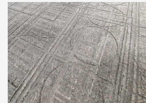
Example of too deep cutting depth
