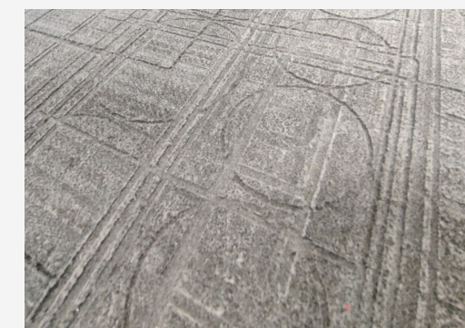
Example of too deep cutting depth
